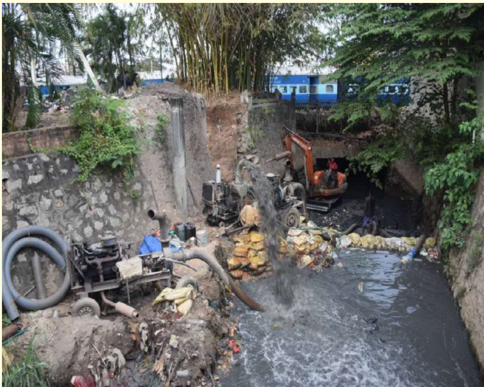
Figure 17 The level difference at the outlet of 140 m Box culvert
