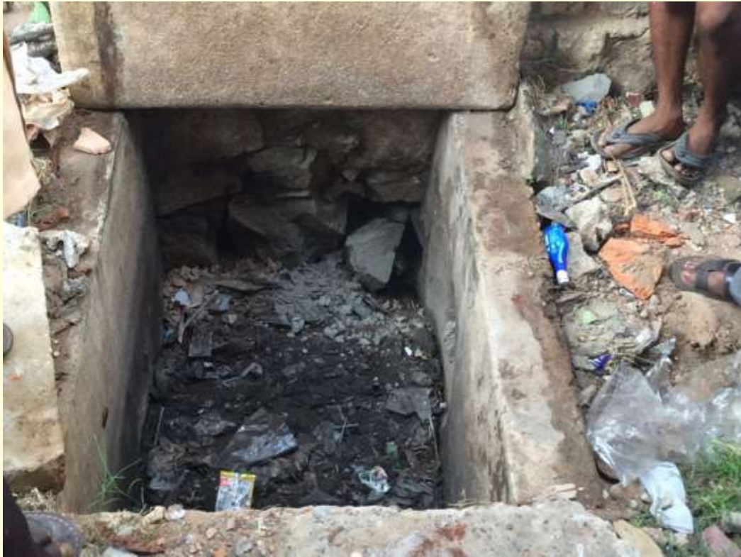
Figure 9 Blocked drains due to foundations of buildings inside drain
