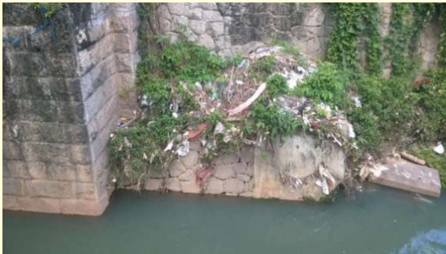
Figure 19 protruded abutment at Uppliamoodu
