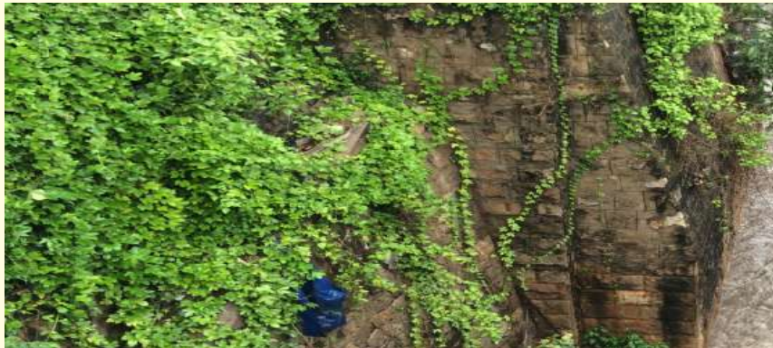
Figure 18 protruded abutment at Uppliamoodu
