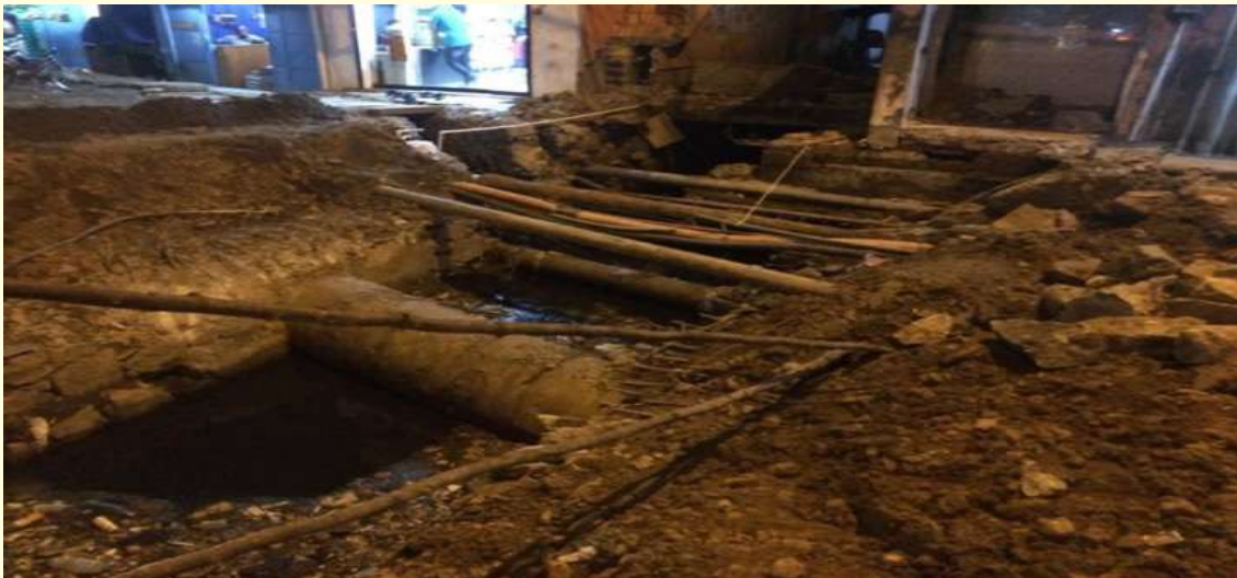
Figure 13 Pipe lines crossing drains at attackulangara
